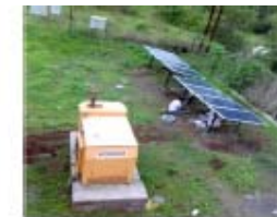
Ground Based Solar Panels
