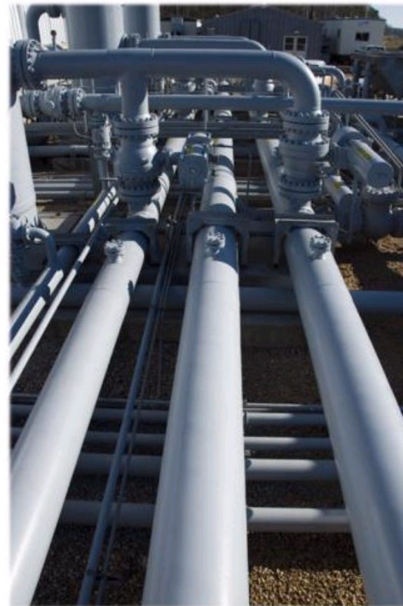
Carthage Compressor Station - Carthage, Texas
